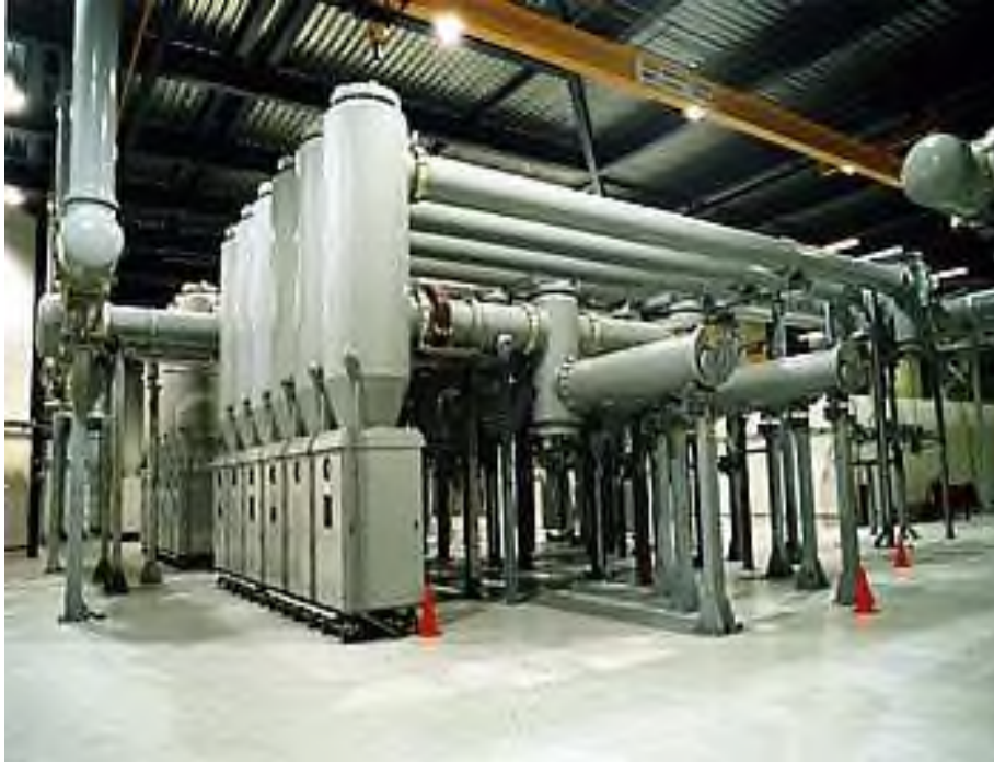
Gas Insulated Switchgear (GIS)
