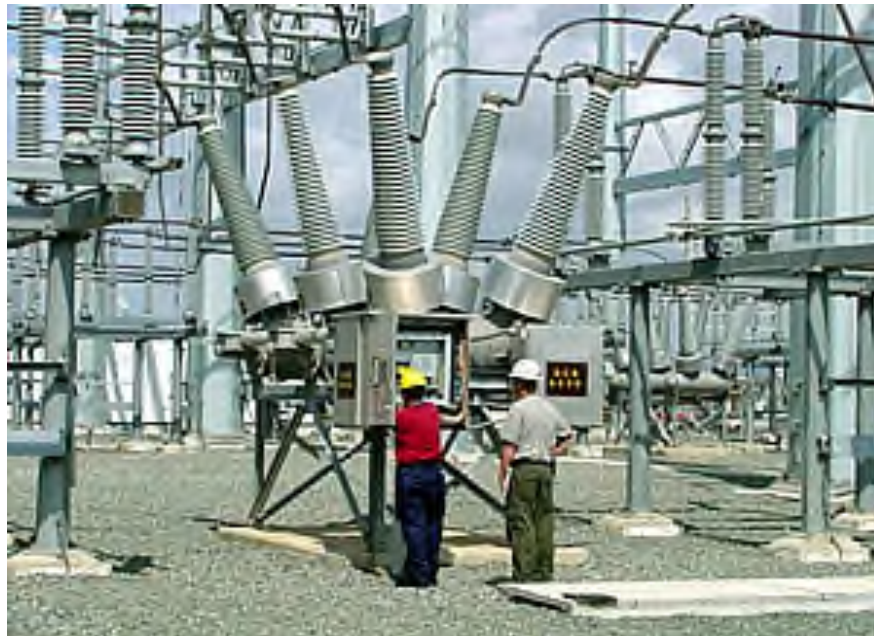
Gas Insulated Switchgear (GIS)
