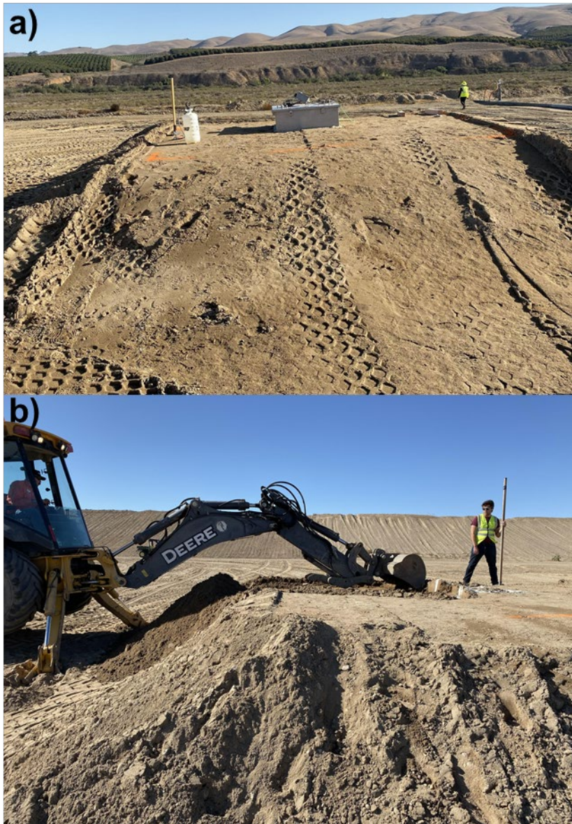
Figure 3.25 a) Static Flux Chamber Testing on the Test Plot Constructed at SMRL, b) Removal of 0.3 m-thick Soil Layer for Testing the Next Cover Thickness.
