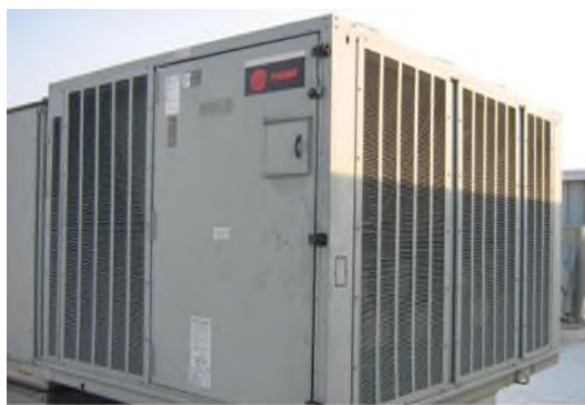
Rooftop HVAC system
