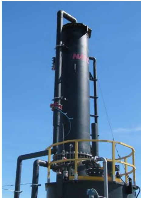
Dairy gas cleanup system (gas scrubber)
