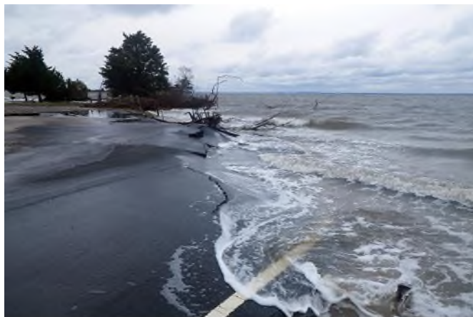
Flood damage from Hurricane Sandy at Assateague Island National Seashore Park (Virginia)
